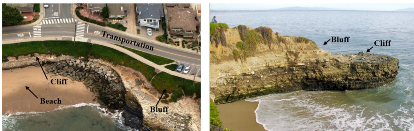
Figure 10-1. West Cliff Drive areas considered for coastal adaptation include the beaches, cliffs, and bluffs; while transportation strategies focus on the cliff top roadway and Recreational Trail (left), coastal adaptation strategies focus on reducing erosion to the hard cliffs and soft bluffs (right).
