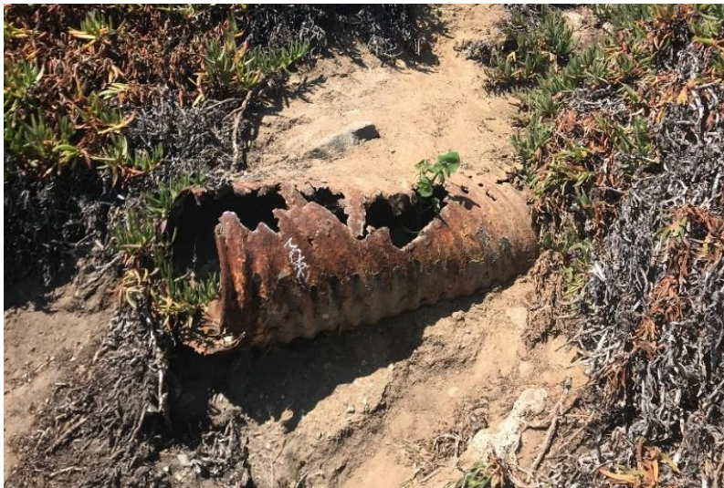
Figure 60. A storm drain outfall along West Cliff in very poor condition
