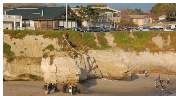
Figure 35. Loss of beach area at Its Beach due to King Tide in Jan 2020 (top), Wave overtopping of the Esplanade wall in Capitola Village during a storm event (middle), cliff erosion along West Cliff (bottom).
