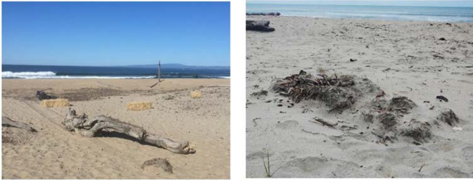
Figure 3. Installation of drift wood and hay bales along the foredune help capture sand and increase dune roughness. Credit: SRSB Dune Restoration Project Final Restoration and Monitoring Report
