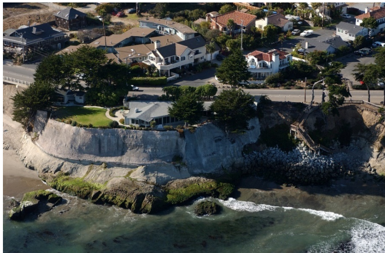
Figure 4: Hard infrastructure mimicking existing cliff face at The Hook, Capitola, California Coastal Records Project. Copyright © 2005 Kenneth & Gabrielle Adelman. All rights reserved.
