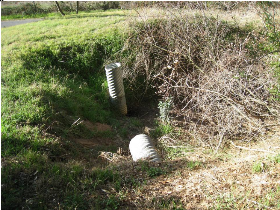
Figure 14 The horizontal culvert brings water from the road into the collecting basin which then flows into the vertical pipe and from here directly into Wagner pond. Before this project, the culvert ended at the edge of Walker Valley Road causing erosion and road flooding
