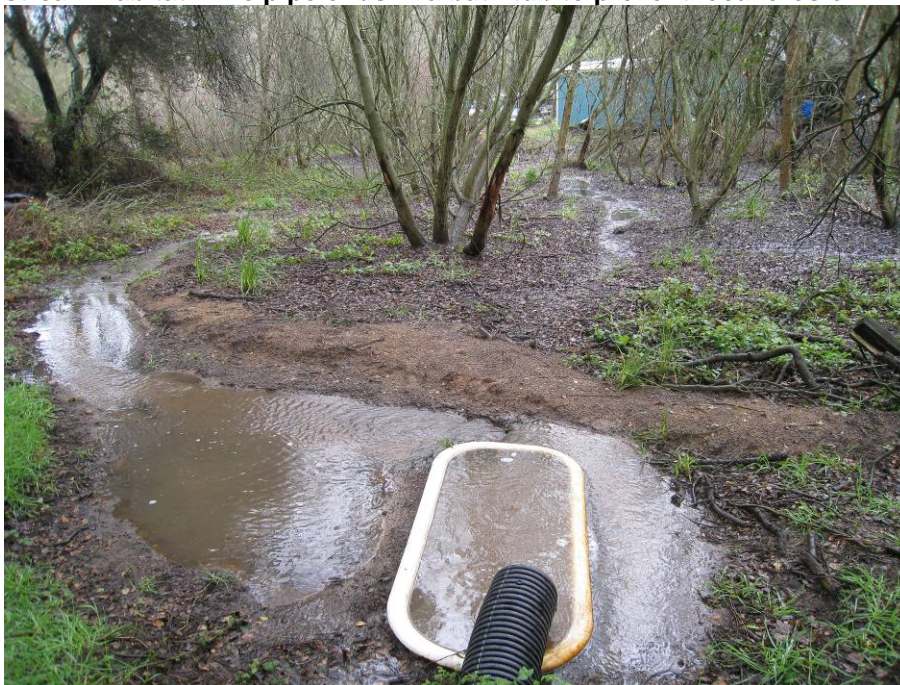
Figure 32 Water enters the upper end of the Guerrero wetland much like it does to Wagner pond, it is collected into a central culvert and piped underground to the top of the natural stream habitat. The pipe ends in a bath tub to prevent local erosion.
