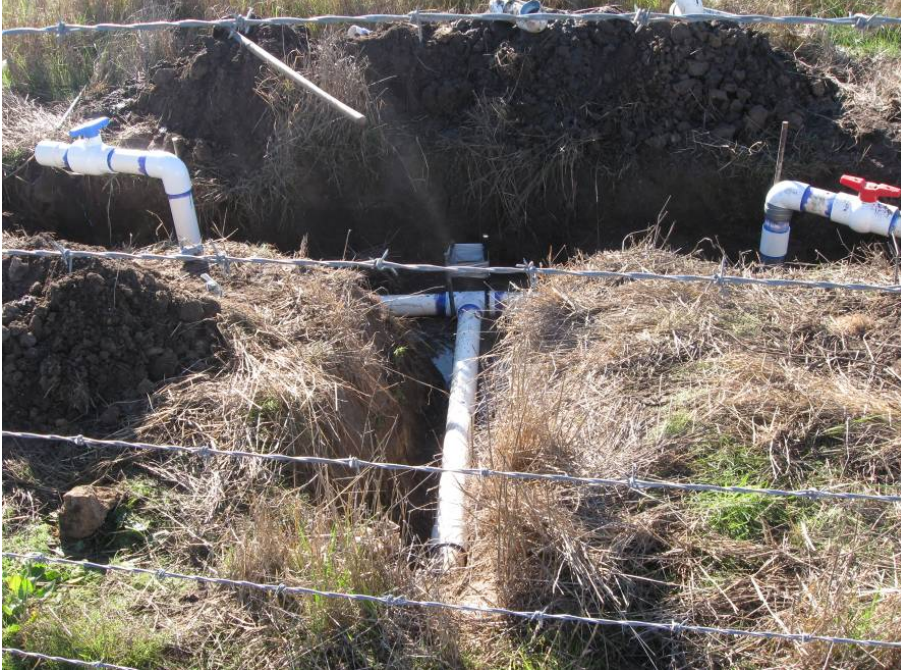
Figure 48 Photograph of new irrigation line being attached to existing line on the slough side
